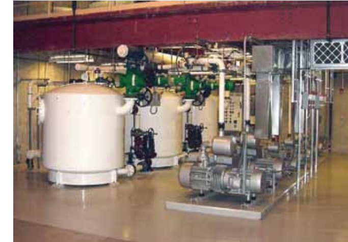
Large Vacuum Tank Assembly
